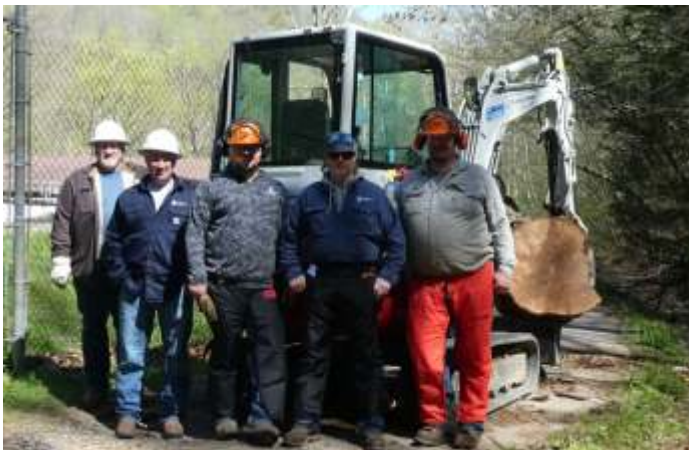
This crew removed the large log from the stream. It took four truck loads to remove the log.
