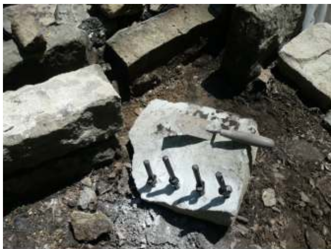
Splitting wedges placed in holes to cut replacement stone for the ring.
